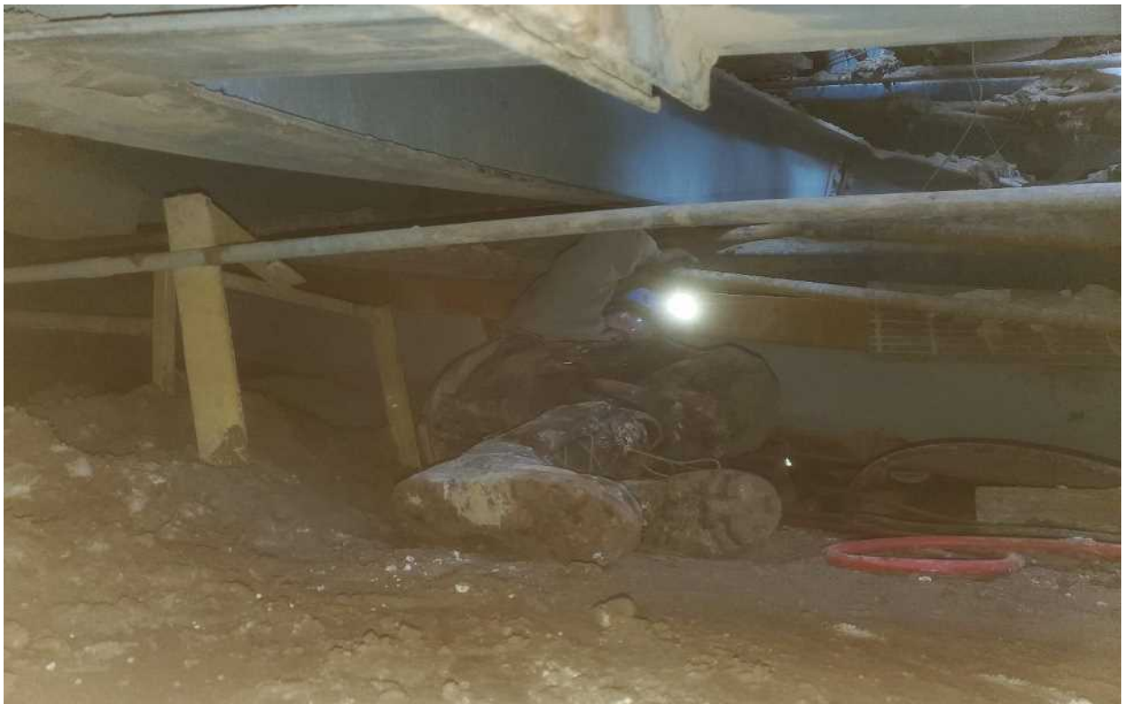
Area of trapped worker
