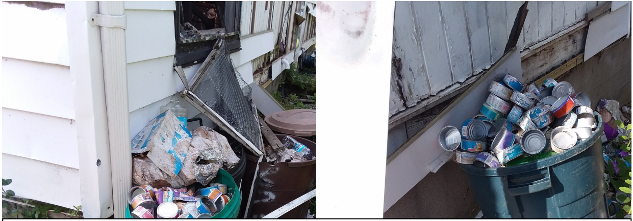
Cat food tins/garbage stored improperly on property – EK – 7/2/19
