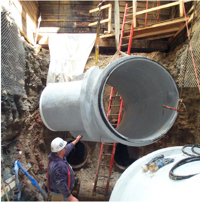
Elsinore Water Main
