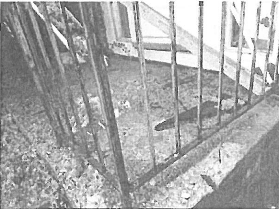
Insulation fallen onto the front porch – EK – 6/17/19
