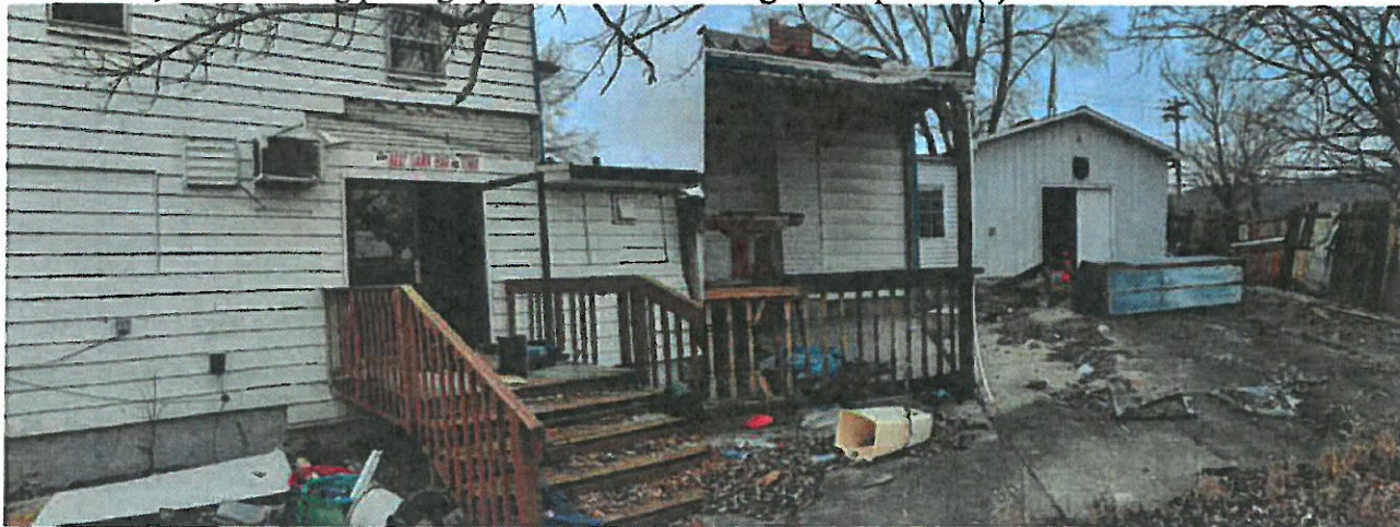
1/28/22 Observed unsecured buildings and debris inside and out of facility. ATB
