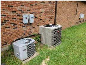
Outdoor Condensing Units
