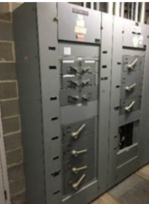
Power Distribution Panelboard
