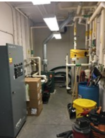
Main Electrical Room
