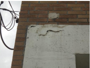
Conc. Portal at door cracking
