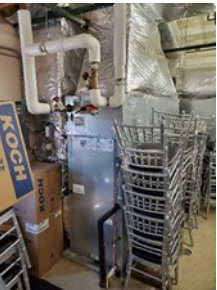
Air Handlers in Mech Room
