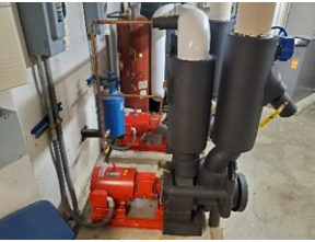
Chilled Water Pump
