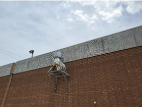
Vehicle Extraction System Fan
