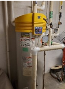
Water Heater & Recirc Pump
