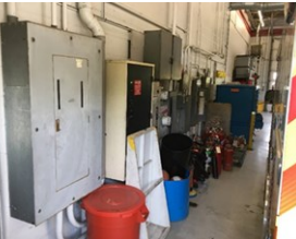
Electrical Equipment in Garage Bay
