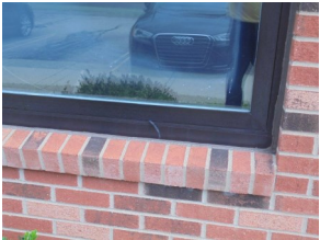
Damaged Window Seal
