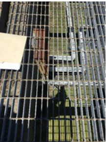
Outdoor Condensing Units in Pit
