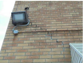
Brick cracking at window
