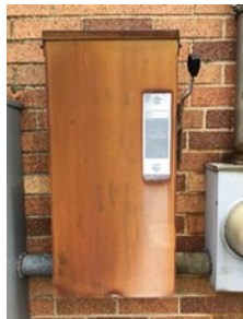
Service Disconnect Switch
