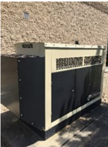
Natural Gas Generator
