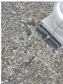
Membrane “Popping” Above Ballast
