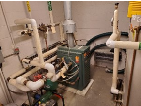
Snow Melt/Radiant Heat Boiler
