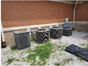
Outdoor Condensing Units
