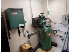
General Service Air Compressor
