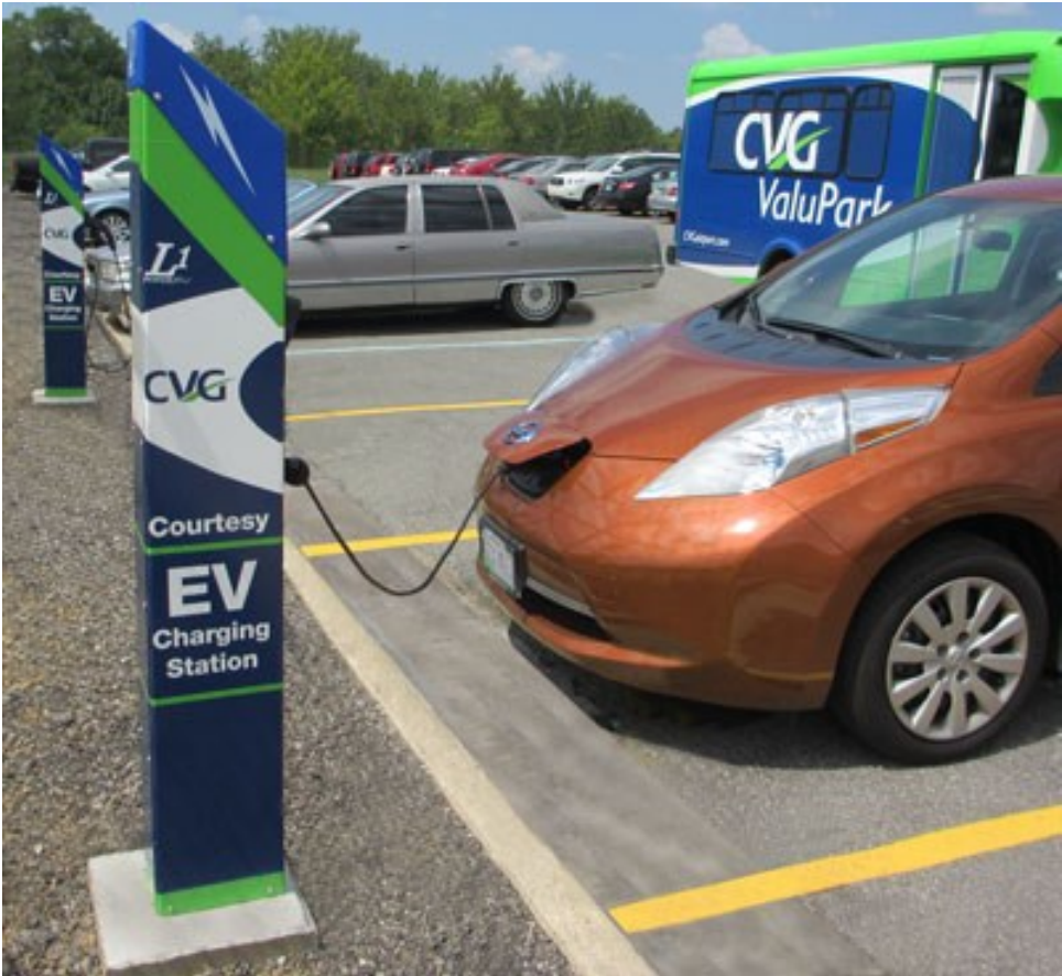
CVG Airport Electric Vehicle Charging Stations - CVG Airport
