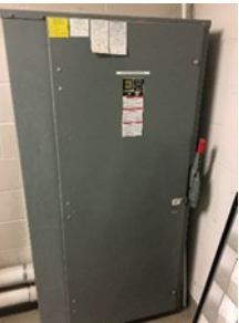
Main Service Disconnect Switch
