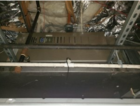
Typ. Horizontal Furnace
