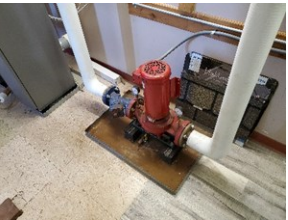
Hot Water Pump
