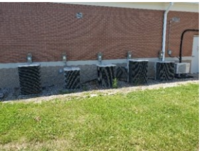
Outdoor Condensing Units
