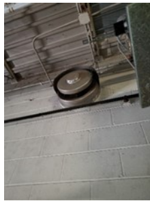
Fan Between Garage Bays
