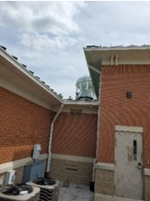
Bay Ventilation Fan (On Roof)
