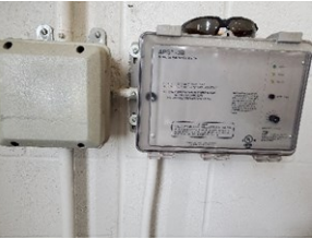
Snow Melt/Radiant Heat Control System
