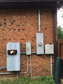
Service Disconnect & ATS
