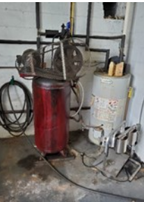
Water Heater (Right)
