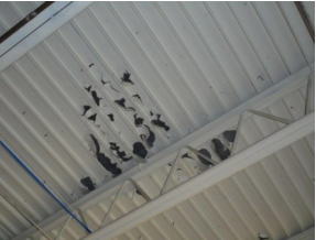
Peeling paint at roof deck
