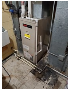
Typ. Vertical Furnace
