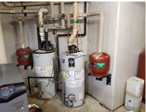
Water Heater and Expansion Tanks
