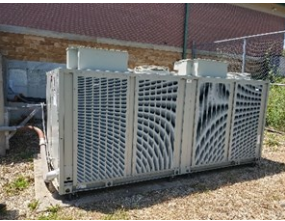
Outdoor Chiller Condenser
