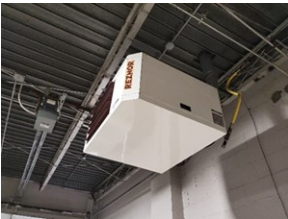
Unit Heater in East Garage
