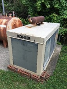
Natural Gas Generator
