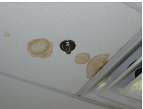
Stained Tile Needs Further Investigation
