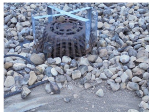
Membrane Not Sealed at Lap Near Drain
