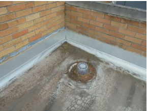
Debris at roof drain
