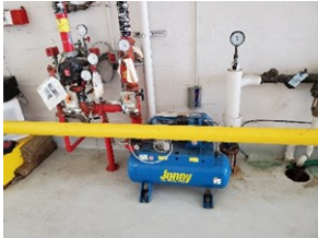
Fire System Air Compressor
