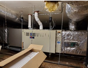
Typ. Horizontal Furnace
