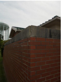
Wall Cap Splitting
