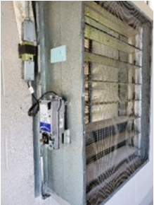
Bay Ventilation Intake Damper
