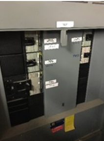
Main Distribution Panelboard
