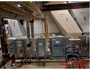
Typ. Basement Air Handler
