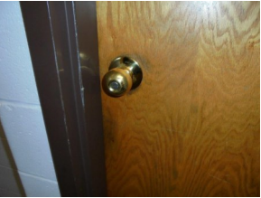
Non-compliant Door Hardware
