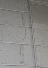
Interior CMU cracking
