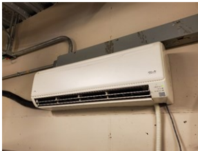
Split System AC Unit in Server Room
