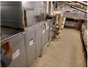
Typ. Attic Air Handler
