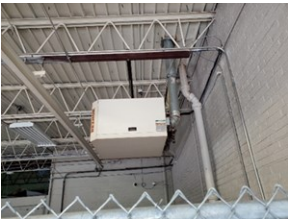
Unit Heater in West Garage
