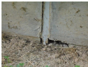
Degraded Wall Base Transition
