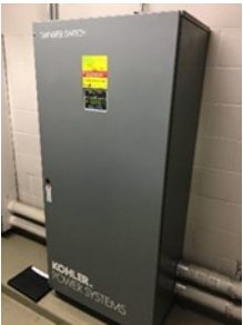
Automatic Transfer Switch
