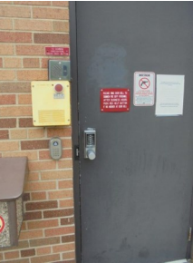
Non-Compliant Door Hardware
