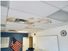
Stains from dripping horiz. ceiling units before pans were installed
