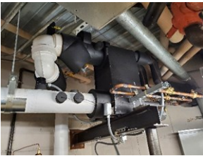
Indoor Chiller Evaporator HX
