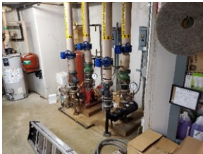
Hot Water Pumps
