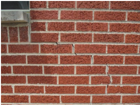
Brick cracking at windows
