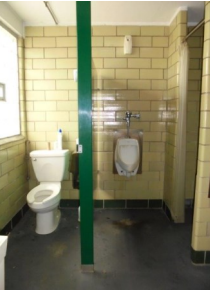
Typ. Restroom fixtures
