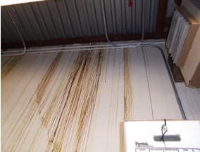
Water Stains on Interior of Wall
