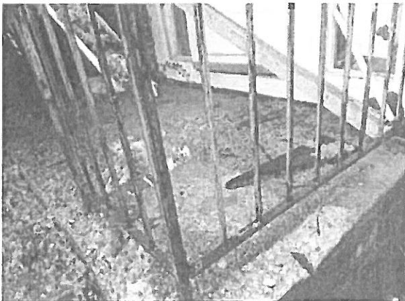
Insulation fallen onto the front porch – EK – 6/17/19
